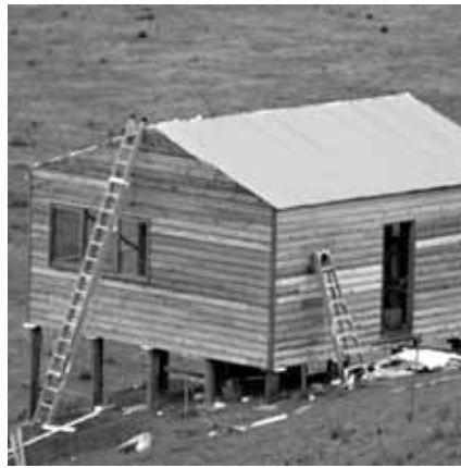
Above left: Colorbond roof, foil backed insulation blanket and polyester batts. Above: Western red cedar cladding to finish.
